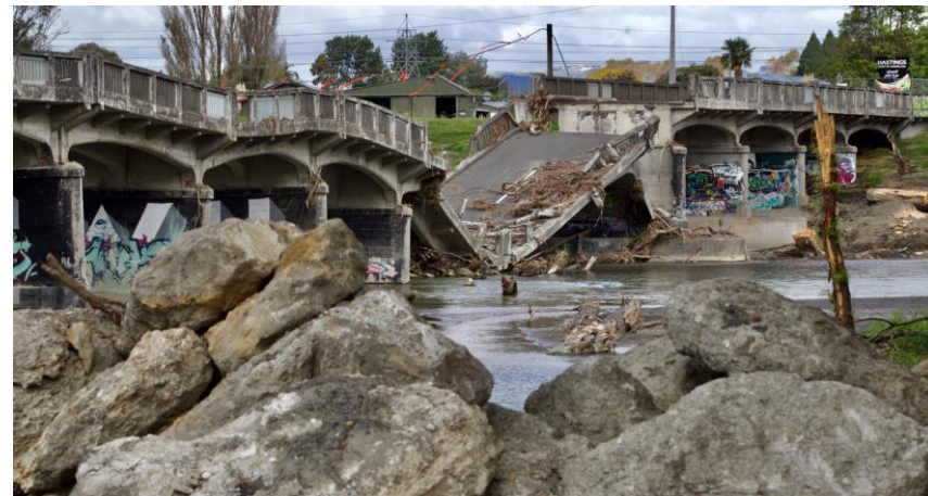
Source Damaged bridge in the Hawke's Bay after Cyclone Gabrielle, February 2023. Photo courtesy of NZ Herald.
